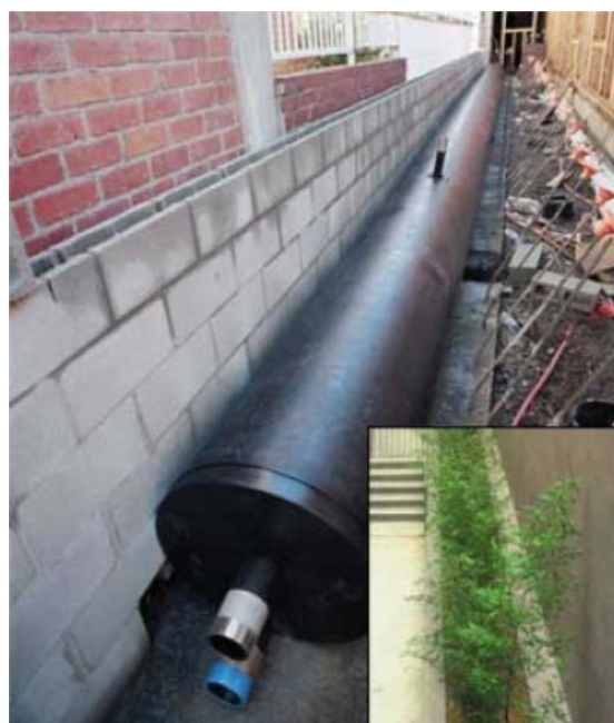
Figure 3-14. Rainwater Cistern at NRDC's Santa Monica Office. (Photo: NRDC) (Used by permission of NRDC)
