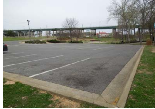
Asphalt pavement with oil and grease stains
