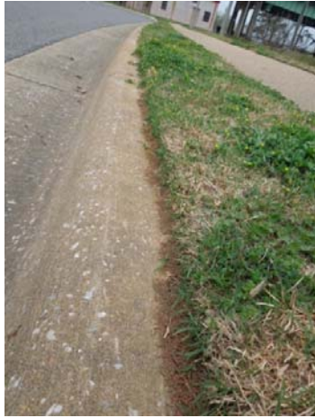
Eroding soils beside the roadway near the filter inlet due to fire ant activity
